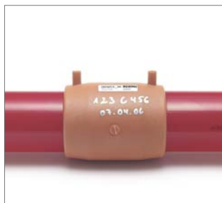
Fig. 108 Using a marker pen, note your personal ID no. and the current date on the electrofusion fitting.
