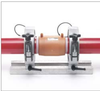
Fig. 99 Prepare the second pipe end, then slide it completely into the electrofusion fitting and secure it with pipe clamps.
