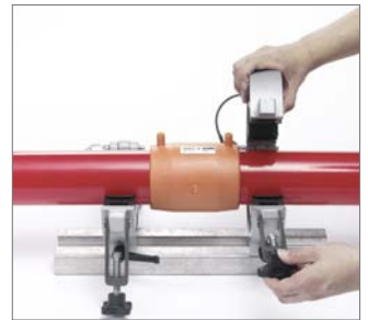
Fig. 106 At the conclusion of the "Cool: ... min." time indicated on the fitting, the universal pipe clamp can be removed.
